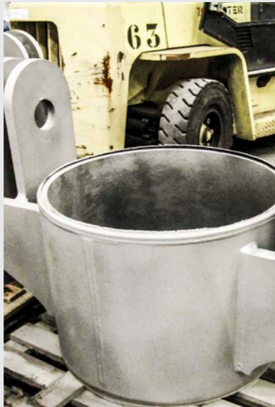
5. Sand blasting of connection ends and hardware that is to be reused. Further preparation for welding.
